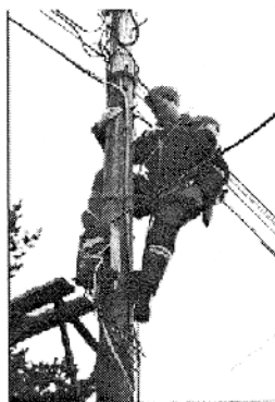
Figure 2: A service engineer at a post.
